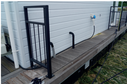
Waste is discharged from the Sanibest Pro in each lodge via 50mm pipework that is routed under the service covers of the pontoon
