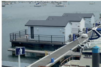
The waste from each lodge runs along the pontoon and discharges into pipework attached to the Saniflos 280
